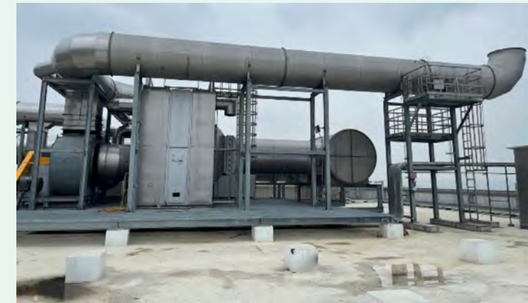
Zeolite rotor and thermal oxidation furnace (TO)
