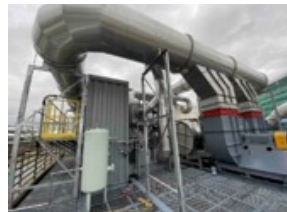
Zeolite wheel and regenerative thermal oxidation furnace (RTO)
