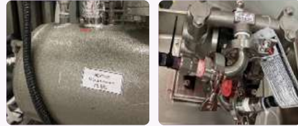
To reduce the escape risk, raw materials are in the liquid state and solvents are transferred through pipelines
