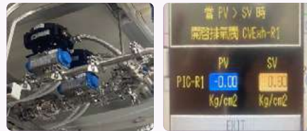
PLC control enables automatic exhaust when the pressure is too high and prevents the vacuum valve and exhaust valve from opening at the same time.
