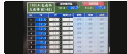
PLC's HMI system features timing and temperature control functions and enables immediate tripping and warning.
