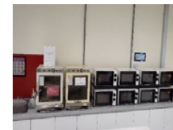
Installed microwaves and electrical appliances
