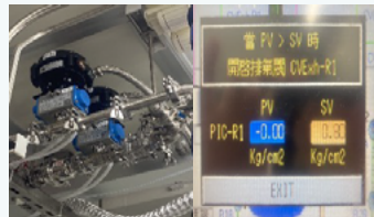
PLC-controlled system with automatic pressure release and simultaneous opening of vacuum and exhaust valves in case of excessive pressure
