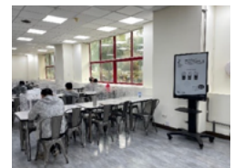
Installed ePaper signage in rest areas
