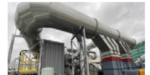
Zeolite wheel + regenerative thermal oxidation furnace (RTO)
