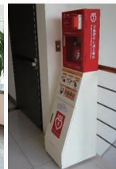
AED setup - Linkou plant
