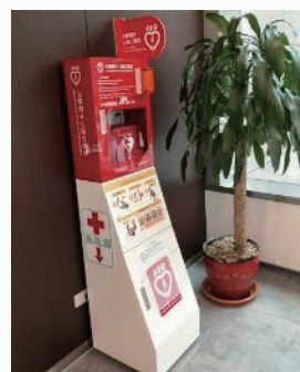
AED setup - Hsinchu plant
