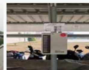
Replacement of power charging station of electric bikes for employees
