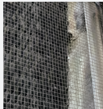
Influence on cooling effect of dirt on cooling materials
